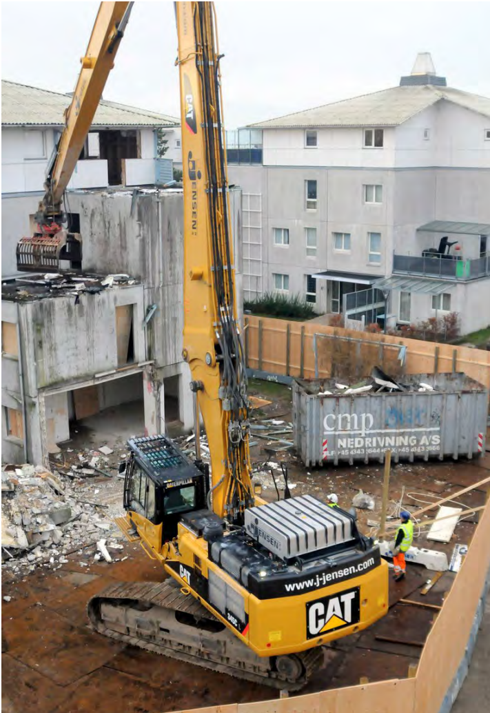
Fig 5 Askerød is one of the few housing areas in Denmark, where some of the buildings were removed in order to obtain a more open area in order to increase the feeling of safety between the buildings. This photo shows the demolition of one of the buildings in 2012. Photo: Greve Nord Projektet.
